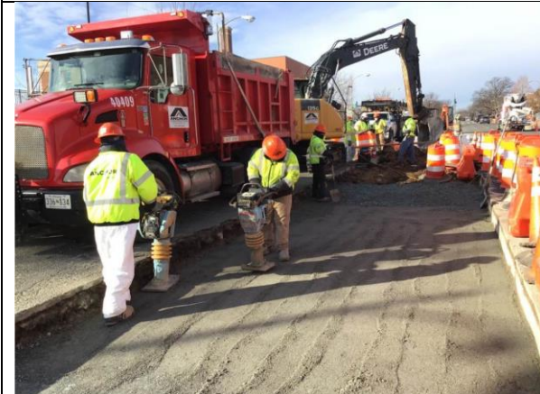
C St NE & 19th – Anchor Place GAB and compact – compaction testing failed
