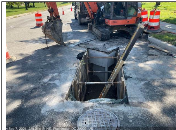
© Sep 7, 2021, 229-21st St NE, Washington DC 20002, US C St NE & 21st St – Excavate 15" RCP between M8-5 to I8-5
