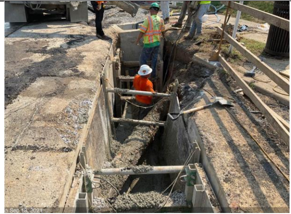
© Sep 13, 2021 C St NE & 19th St – Concrete cradle for 15" RCP between M6-10 to I7-3
