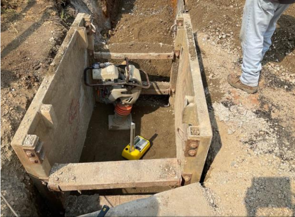
© Sep 14, 2021 C St NE & 19th St – Backfill 15" RCP between M6-10 to I7-3
