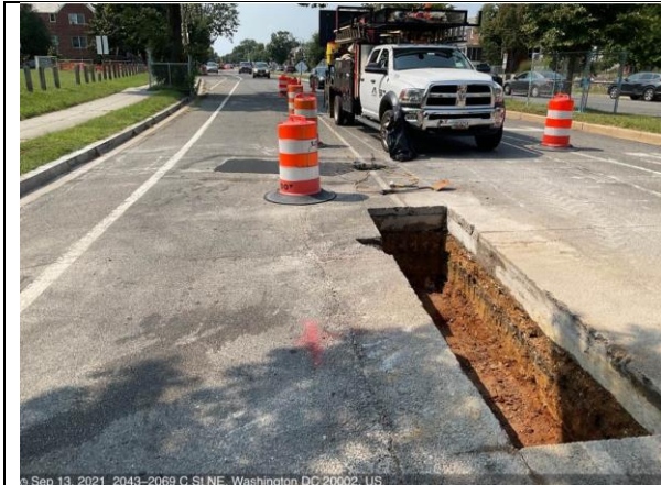
© Sep 13, 2021, 2043-2069 C St NE, Washington DC 20002, US C St NE & 21st St – Test pit for PEPCO facility between M8-2 and I8-2
