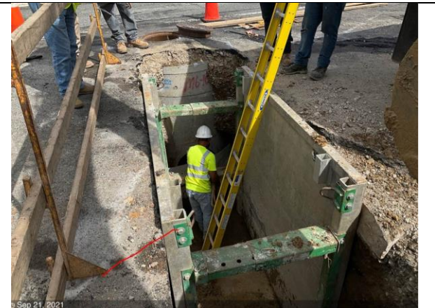
C St NE & 19th – Excavate, for 15" RCP between inlet I6-11 and manhole M6-10
