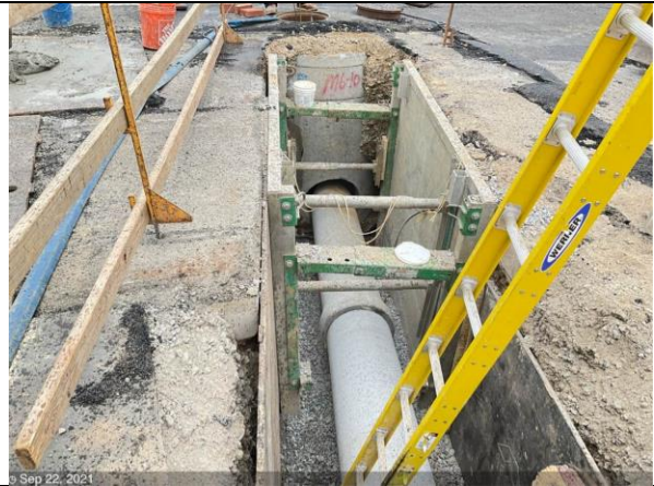
C St NE & 19th – Install 15" RCP between inlet I6-11 and manhole M6-10
