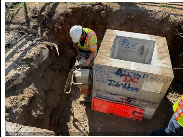
C St NE & 19th St – Excavate, place, and backfill inlet I6-11 with RC-6
