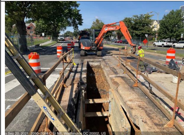
C St NE & 21st St – Trench excavation for 15" RCP between M8-7 and M8-2 (RFI 043)
