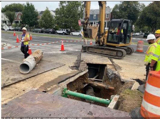
C St NE & 20 th St – M7-4 to I7-12 remove soft material and reset pipe
