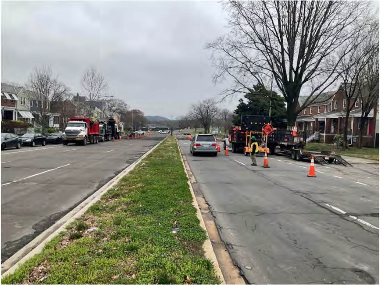
Picture No. 4 – 03252021 – Verizon pavement restoration, C St NE at 20 th , looking west
