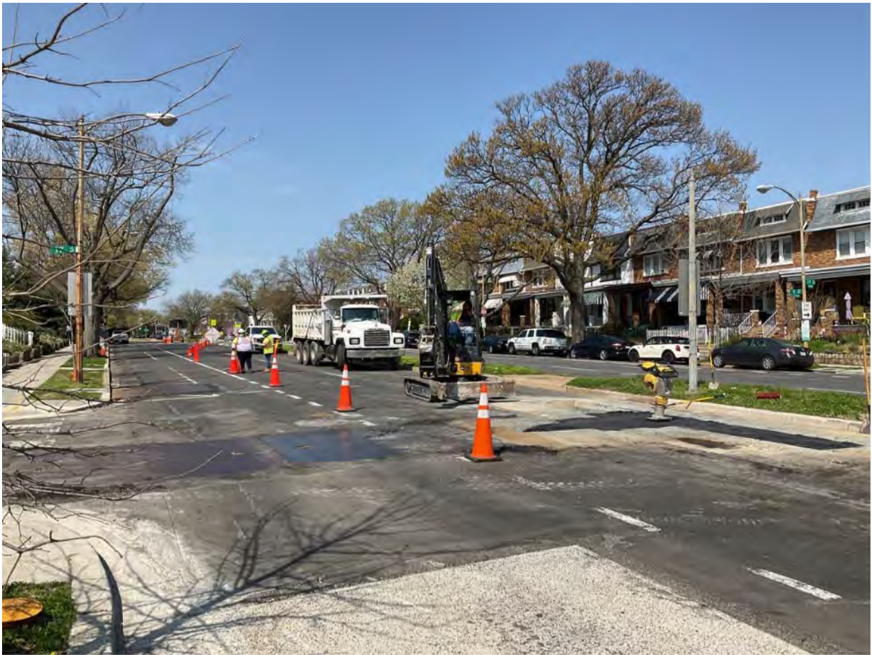
Picture No. 3 – 04062021 – WGL Relocation C St NE & 17 th St PI, looking west
